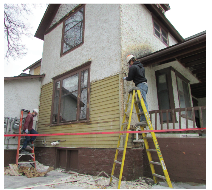
Employees of Trust Thermal take off stucco on the side of the house which was built in 1903 but has been abandoned in recent years.
